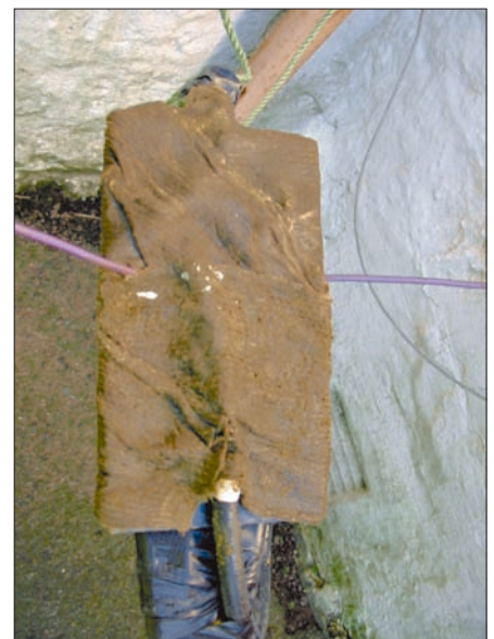
Fig. 5: Waterproofing the centre-piece with sticky Denso Tape keeps the weather out of the joints.
